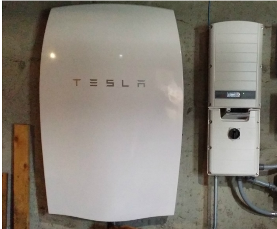
(a) Tesla Powerwall
